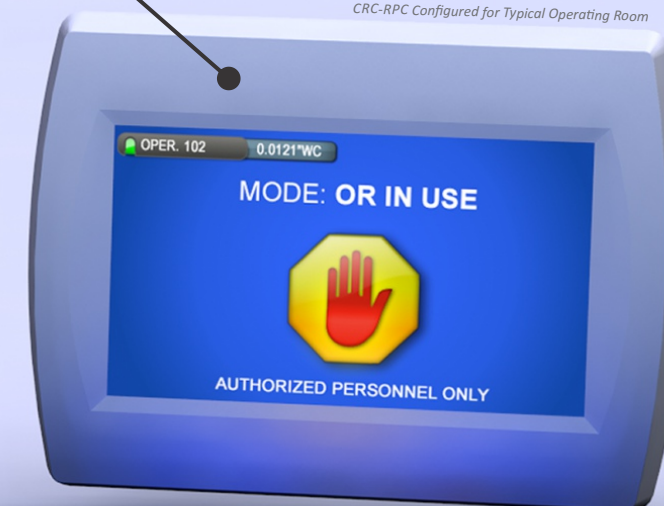
CRC-RPC Configured for Typical Operating Room
